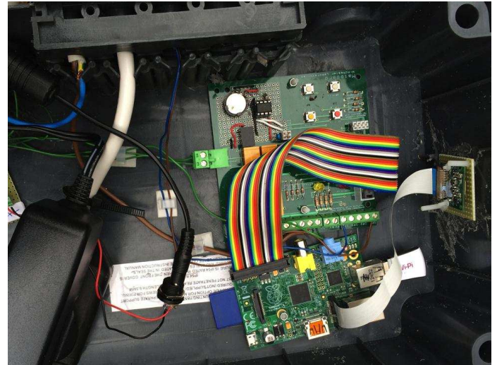
Raspberry Pi and Matboard controlling a water pump
